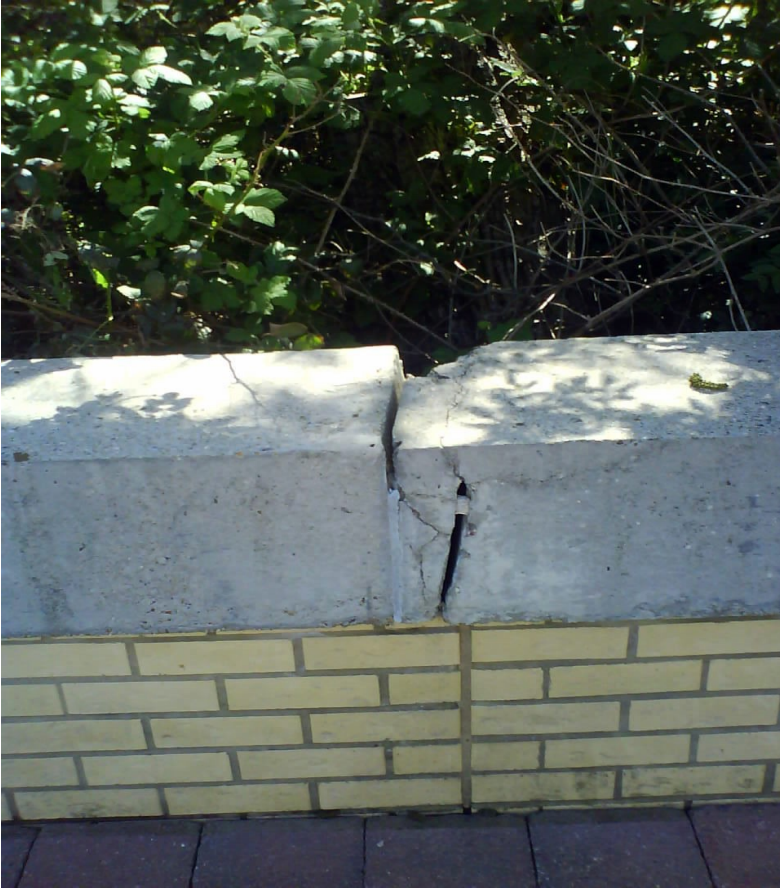
Figure A 19: Extra broadly wall destroyed by tree.
